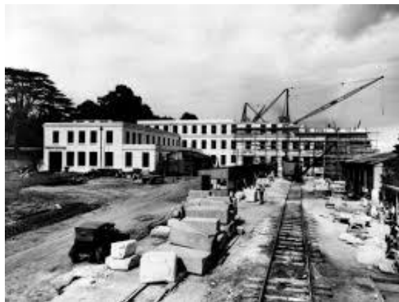
The Trent Building under construction, prior to the iconic clock tower being added.
