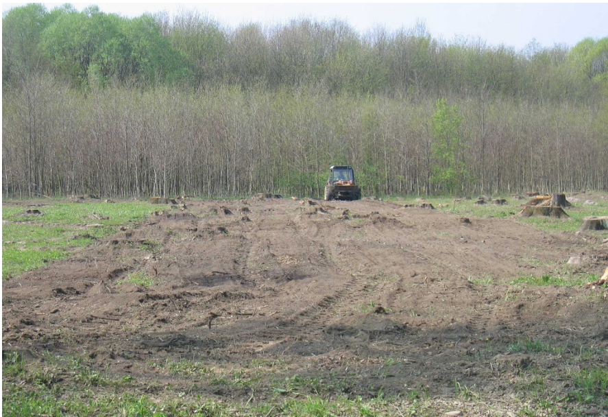
Figure 12. Surface preparation for tree planting in a protected forest area close to Olomouc. Credit: Libor Mazánek.
