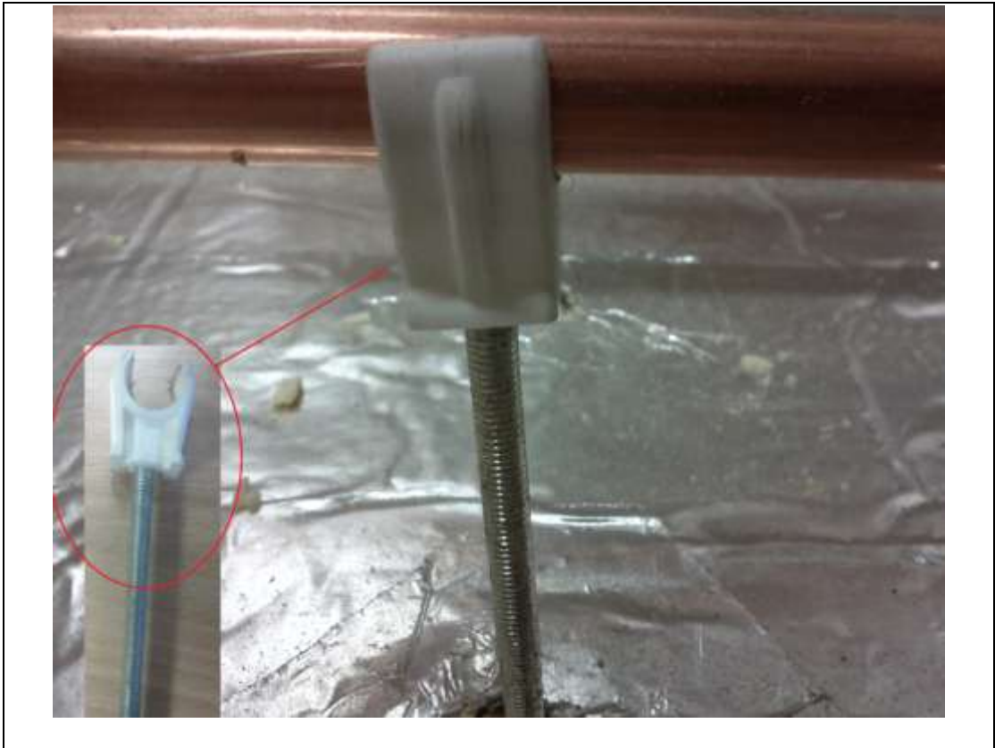
Figure 5-6 Storage pipes rested on supports
